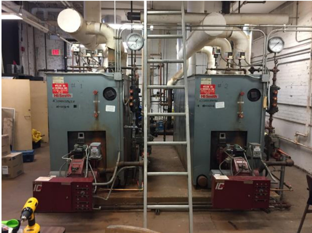
Image 2 – Steam Heating System
